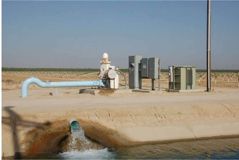
Figure 3.3 Typical Groundwater Well Discharging to a Main Conveyance Canal.
